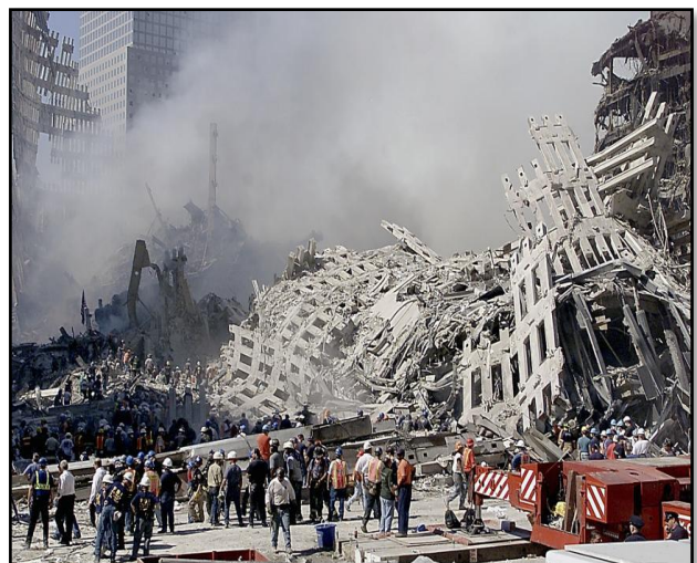
Figure 2. Search, rescue and recovery operation at Ground Zero
